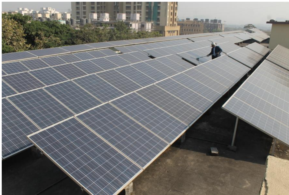
Solar Panels installed on the campus
